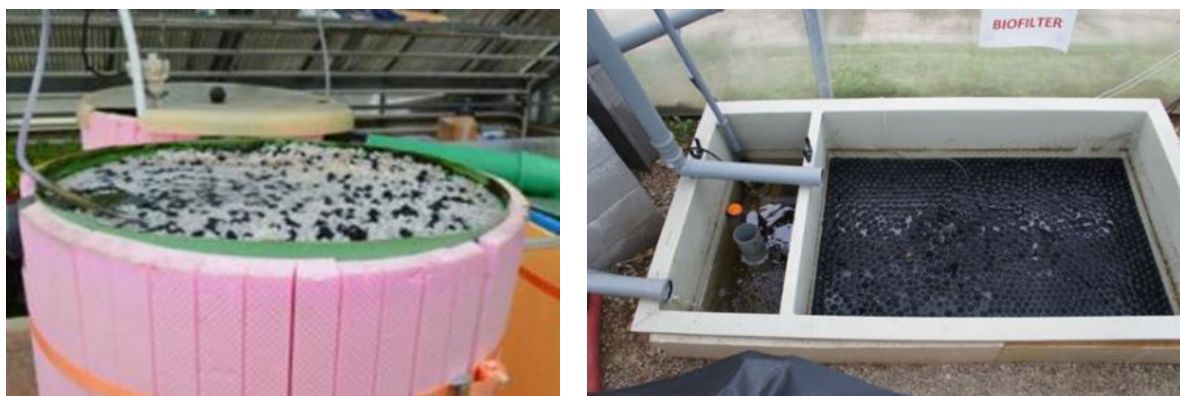
Figure 13: Two versions of suboptimal moving media biofilters: (left) biofilter containing too many biochips (photo R. Bolt); (right) biofilter with no aeration (photo: U. Strniša)
